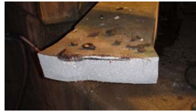
Photo showing broken gate anchorage (USACE photo)
